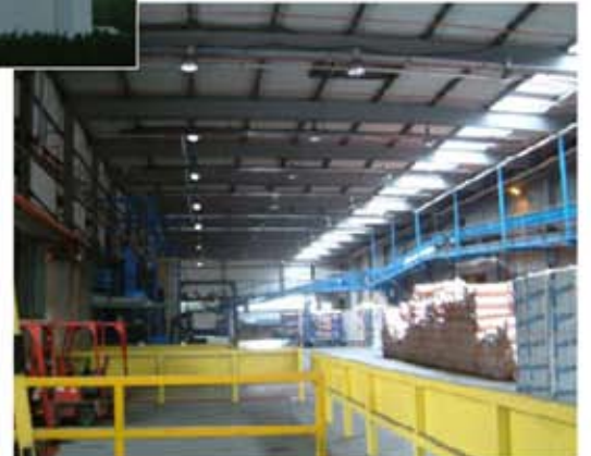
Cooling Bay - 250 Watt Metal Halide
