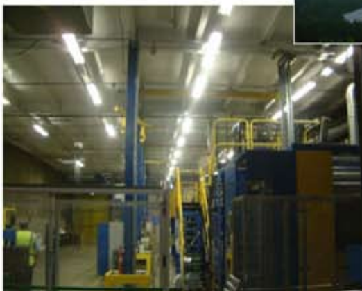
Batch Plant - 6 ft Fluorescent
